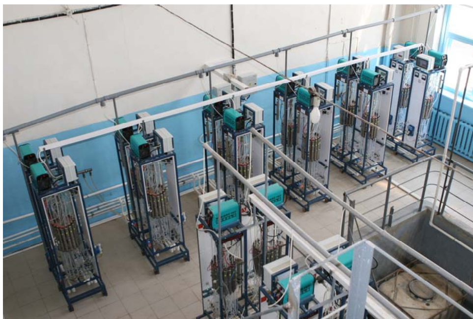
Figure 5. AQUACHLOR-500 devices at water treatment station, Balakovo. There are 76 A-500 devices at station including reserve ones. Daily productivity of system in equivalent of molecular chlorine – more than 900 kg.
